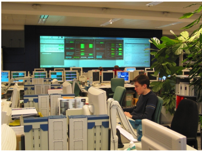
TransVision in a control room
